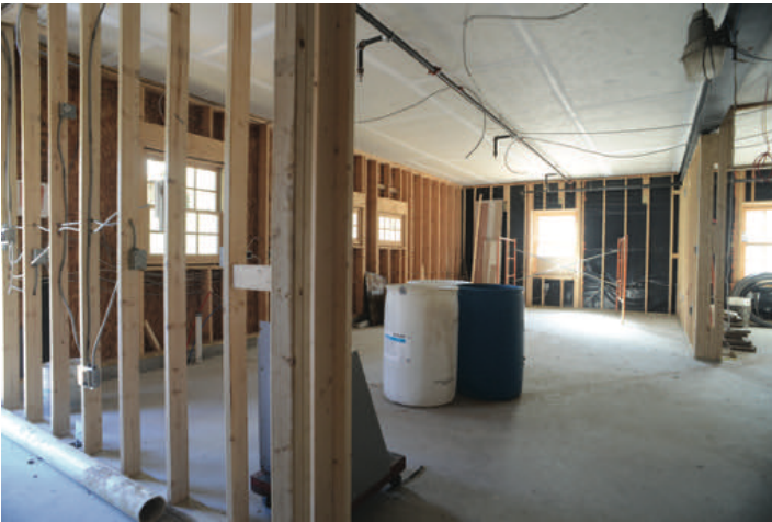
Uncompleted caretaker's apartment and public restrooms in the lower level of the barn.
